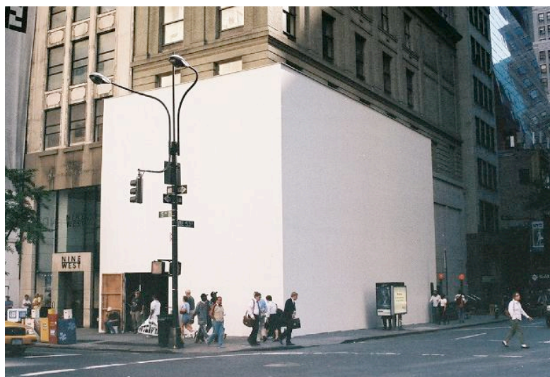
Wall and Scaffolding Installation Corner of 5th Avenue and 53rd Street, New York, NY
